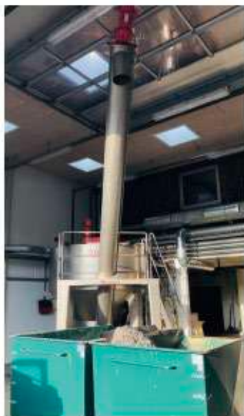
The washed sand is dried by gravity while conveyed directly to a container – ready for transportation and reuse.
